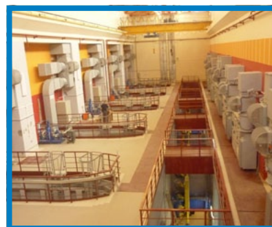
Grodnenskaya HPP Powerhouse Interior
