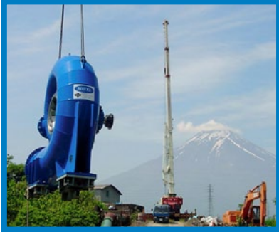
Fujiyoshida HPP / Japan 1 x Francis / 140 kW
