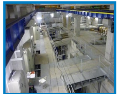
Lovosice HPP Powerhouse Interior
